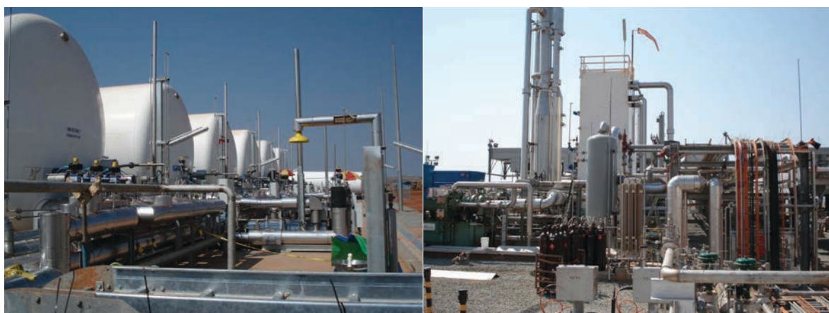
Figure 21. EDL virtual pipeline facility: LNG storage tanks (left) and cold box unit (right).
