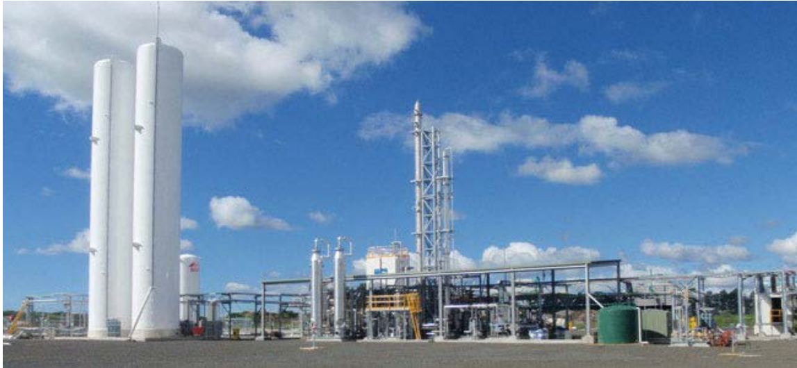
Figure 20. The BOC micro-LNG plant in Westbury, Tasmania.
